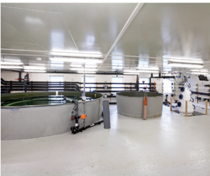
Technical hall with fish tanks and gas-dissolving equipment
